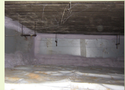
This masonry Pilot unit's crawl space shows spray foam, which the Board is not recommending.
